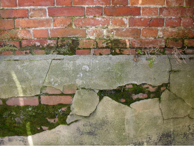
Figure 8: Defects such as damp walls can reduce the thermal performance of the building envelope.
