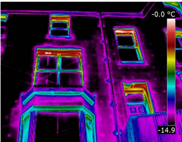
Figure 11: Thermal imaging cameras show variations in surface temperature and can highlight thermal defects such as cold bridges (© Dr Jo Atkinson).
